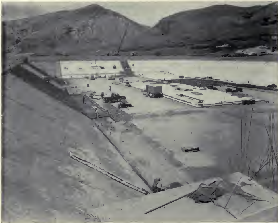
NORTH TERMINAL— Placing concrete in No. 2 (north) reservoir of Salt Lake Aqueduct Terminal Reservoir. Parley's con- yon moyn gateway to the east can be seen in the background.
